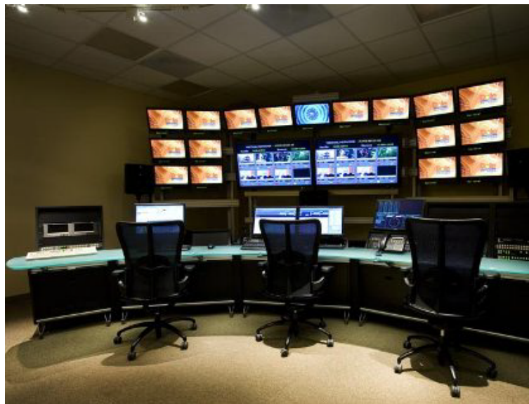
Figure 1 A modern control room [10]
